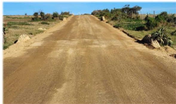
After scraping and compacting of the road ensuring good drainage of the road.
