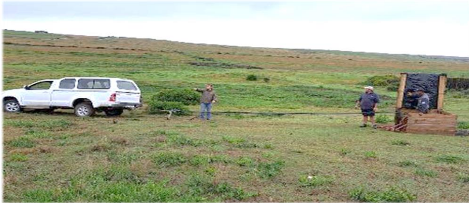
The borehole pump was serviced, and a duty/standby pump arrangement is now in place.
