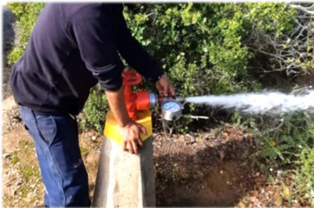
Annual testing of Estate fire hydrants – May 2023
